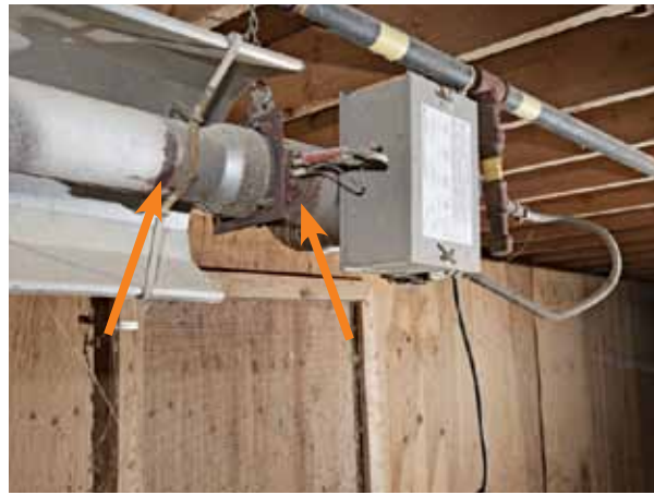
Figure 2.8b. Front view of a radiant tube heater inside the same broiler barn. Corrosion is present.
