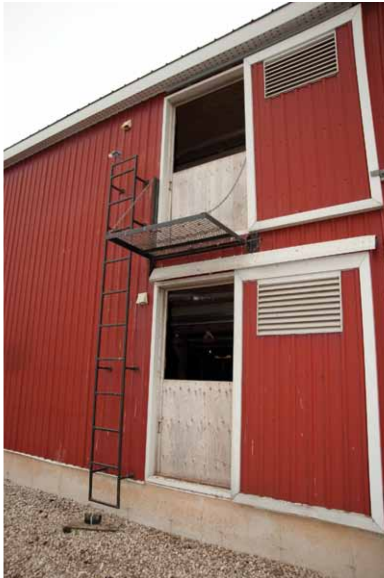
Figure 4.9. An example of a fire exit ladder located beside exit doors on a two storey broiler barn.
