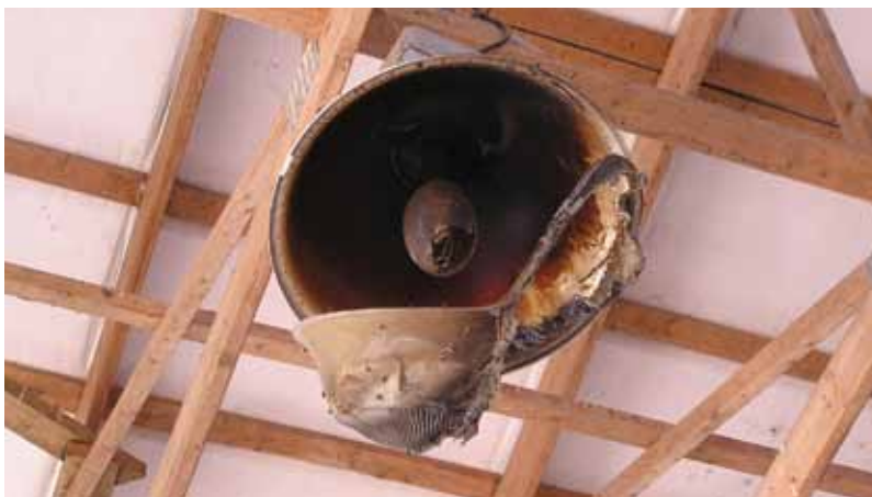
Figure 2.2. Light fixture in a dairy barn that caught fire due to the presence of a bird’s nest (proximity of combustibles). (Photo credit: R. Drysdale, Farm Mutual Reinsurance Plan)
