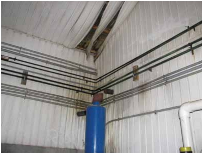
Figure 3.11. Melted vinyl sheathing on ceiling. Note the lack of backing behind the vinyl leaving the attic space exposed.
